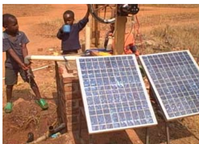
Two children test out the solar powered rope pump in Mzuzu, Malawi. October 2008.
