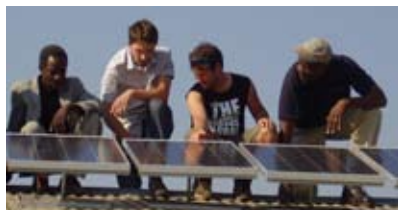
SolarAid Zambia team on the roof of Chilimboyi CABLAC, Zambia
